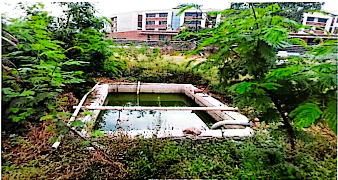
Photo No. 27: Sewage Treatment Plant Facility (A), (B)
