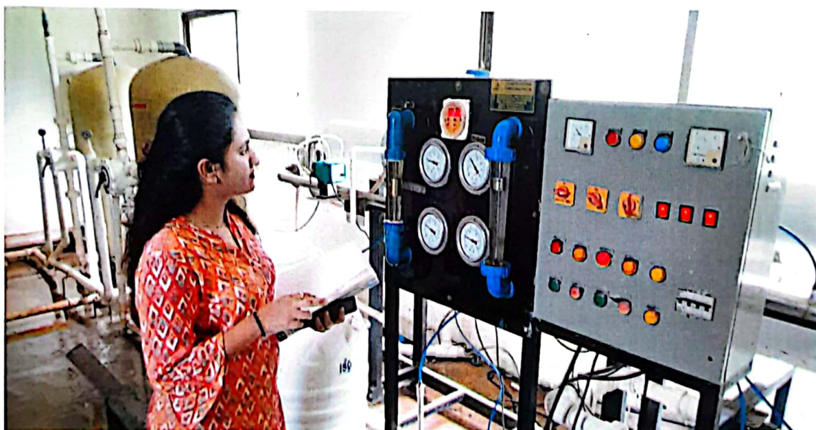
Photo No. 31: Centralized Reverse Osmosis Distribution Facility (A), (B)
