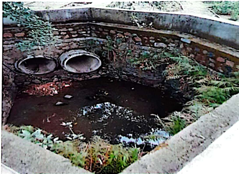
Photo No. 26: Rain water Harvesting (A), (B), (C)
