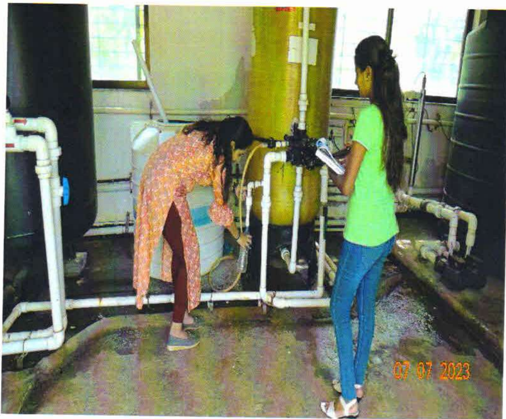
Photo No. 31: Centralized Reverse Osmosis Distribution Facility (A), (B)
