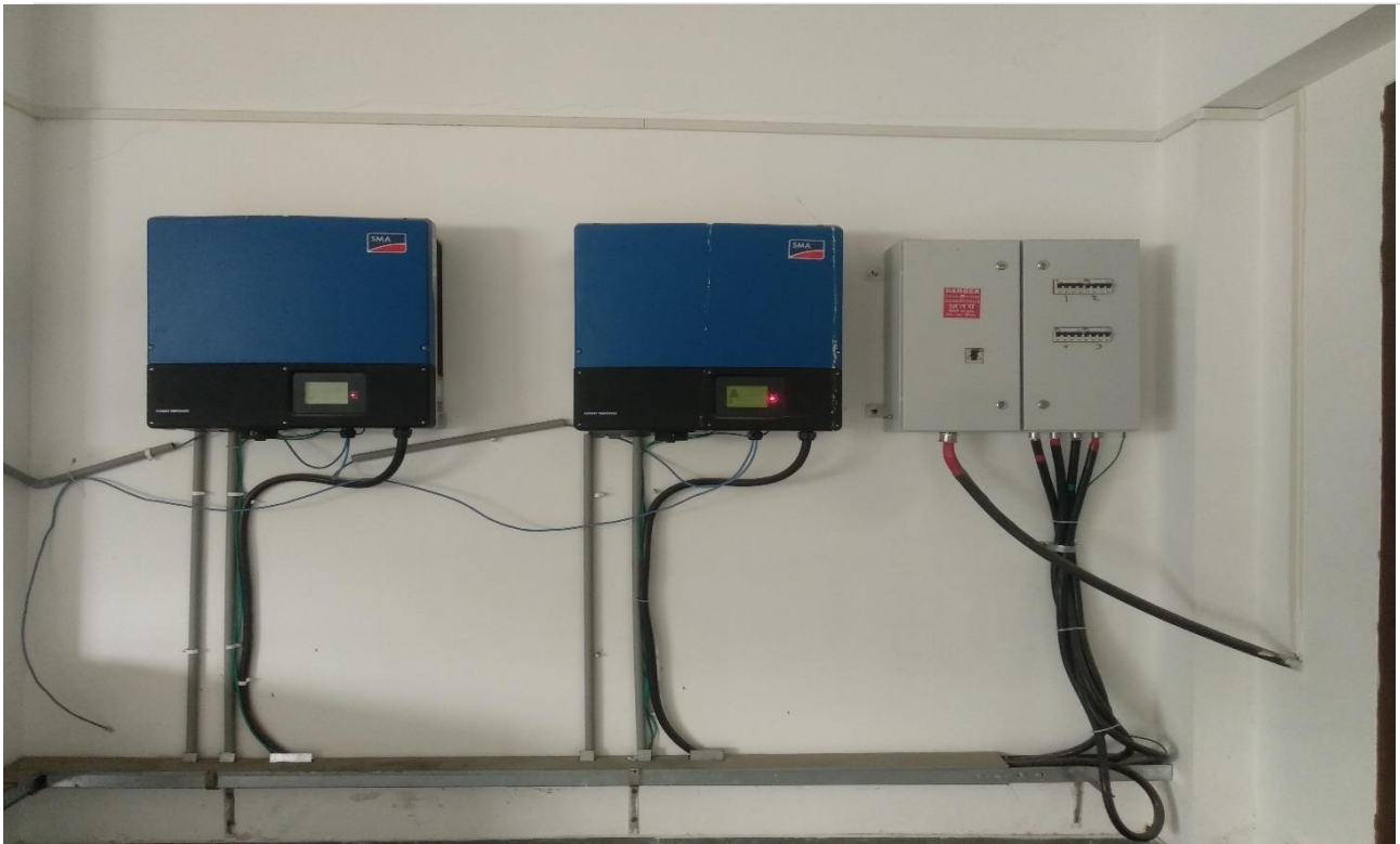
Fig.1. MEDCL Electricity supply facility of SIPS Building
