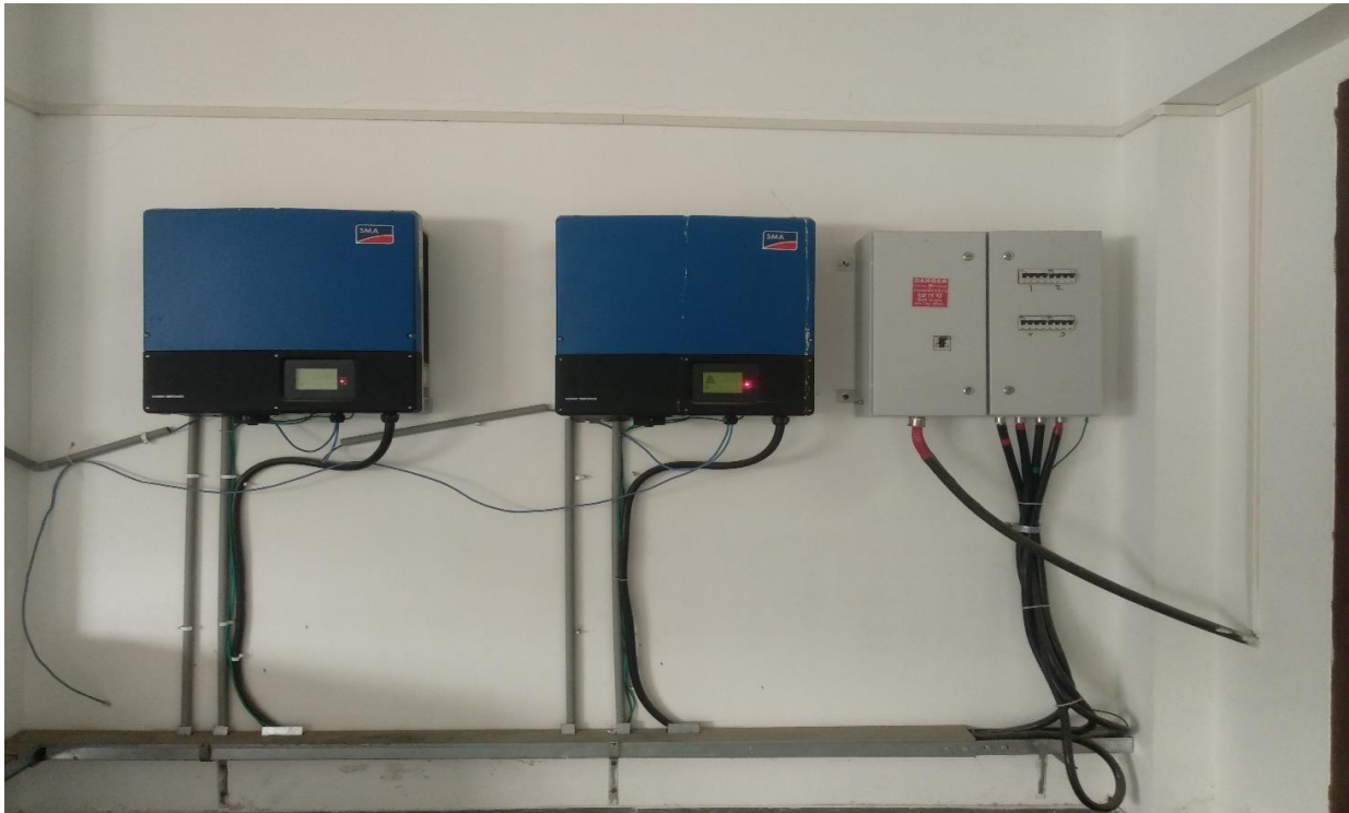
Fig.1. MEDCL Electricity supply facility of SIPS Building
